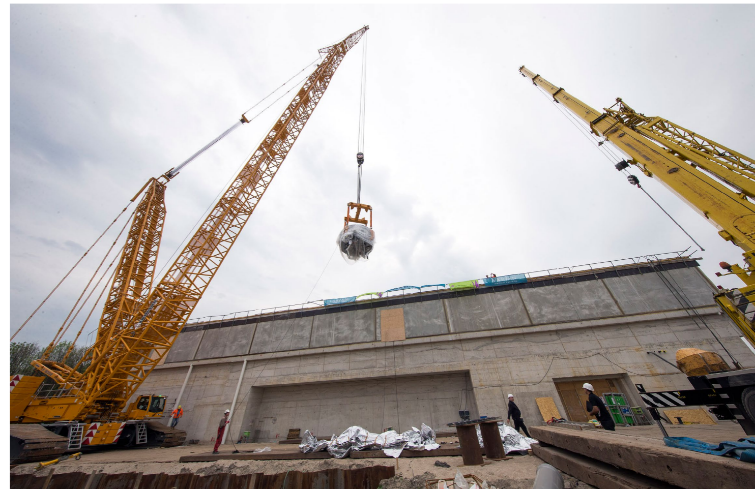
Installation of the cyclotron. © Levien Willemse
