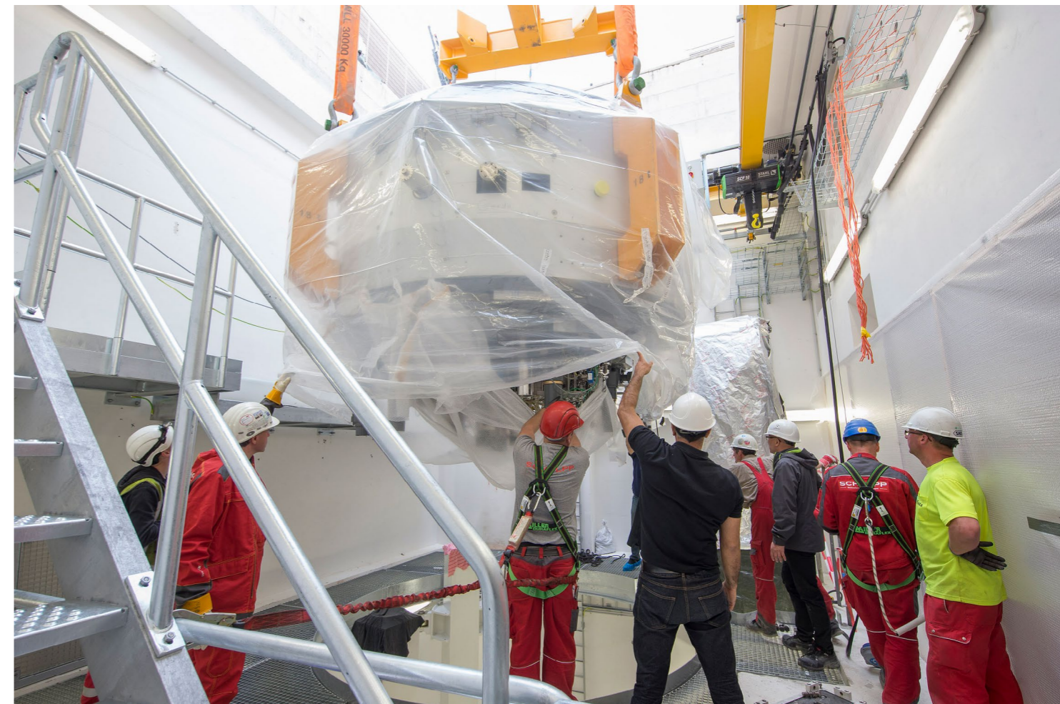
Installation of the cyclotron. © Levien Willemse
