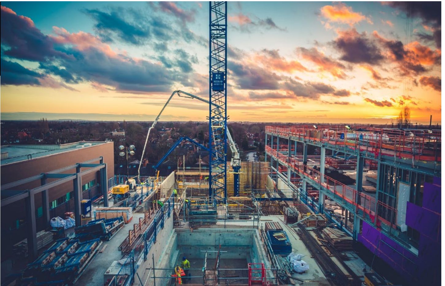
Construction of the clinical proton centre at the Christie (picture taken on Feb 14th 2017)
